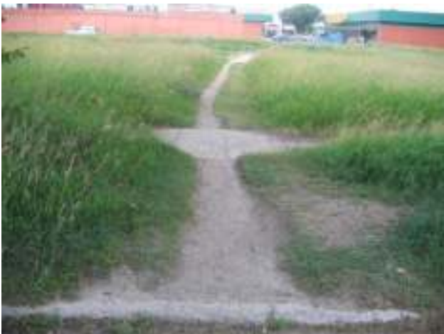
Photo 29: Worn Foot Path North of South Front Street
